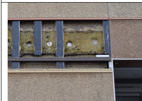
Figure 59: Close up view of compartment floor detail, which shows mineral wool insulation installed at compartment floor location, but this does not fully fill the void behind the Steni GRP rainscreen cladding panel (Taken from Queens Court 2021).
