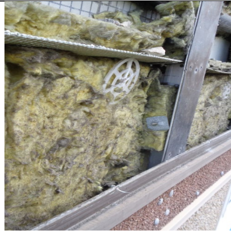
Figure 26: General view of unsuitable vertical cavity barrier installed at compartment wall location – cavity barrier is not in compression against the rear of the Steni GRP panel.
