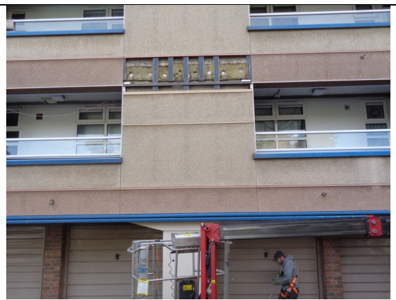
Figure 58: General view of compartment floor location to show no horizontal cavity barrier at compartment (Taken from Queens Court 2021).
