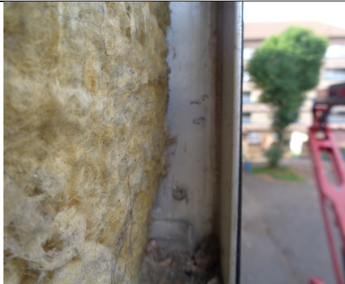
Figure 63: Close up view at compartment floor location to show that the mineral wool insulation does not fully fill the void and therefore does not form a suitable cavity barrier at compartment floor location (Taken from Queens Court 2021)
