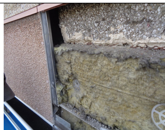
Figure 60: Alternative view of compartment floor detail, which shows mineral wool insulation installed at compartment floor location, but this does not fully fill the void behind the Steni GRP rainscreen cladding panel and the concrete floor slab (Taken from Queens Court 2021).
