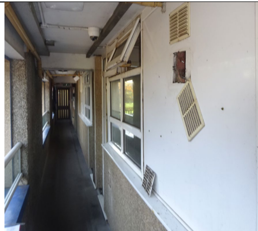
Figure 70: General view of the sample location at first floor level (Harold Court).
