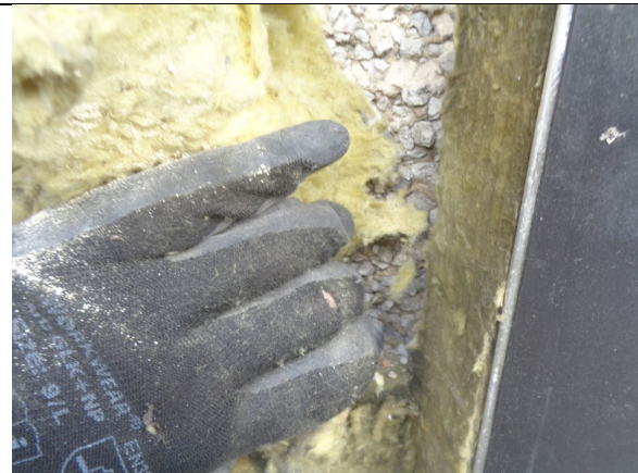
Figure 26: General view of unsuitable vertical cavity barrier installed at compartment wall location – cavity barrier is not in compression against the rear of the Steni GRP panel.
