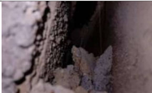
Figure 37: General view to show clear cavity located between inner blockwork lead and outer blockwork leaf.
